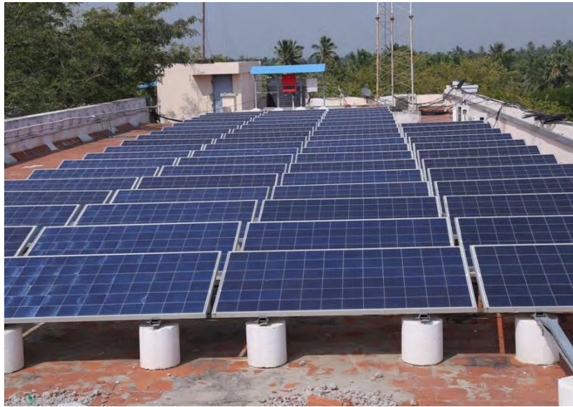
Photo 7: Solar panels installed in top roof
