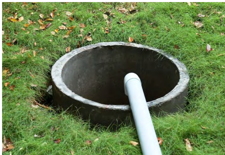
Photo 2: Rain water harvesting system
