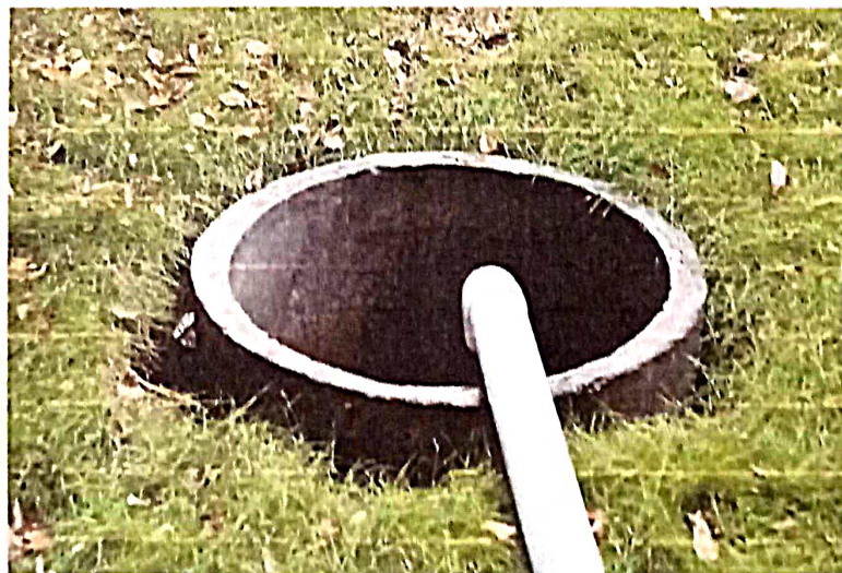
Photo 2: Rain water harvesting system
