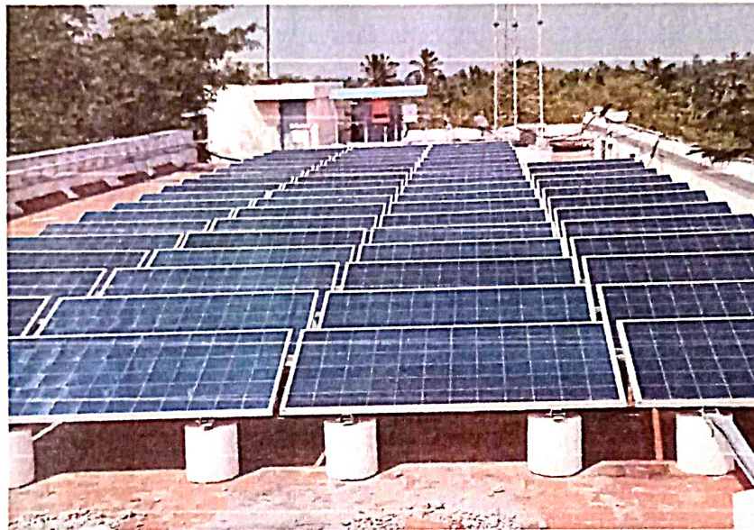
Photo 7: Solar panels installed in top roof
