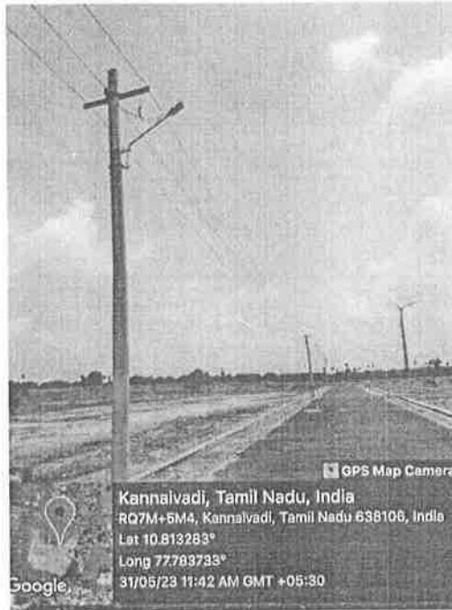
Fig. 5 Street Light provision
